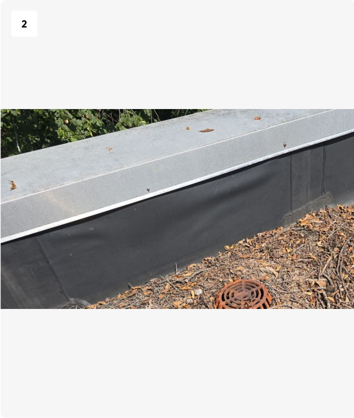
Localized delamination of wall flashing
