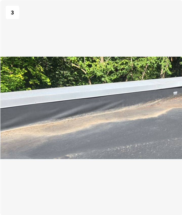
Localized delamination of wall flashing
